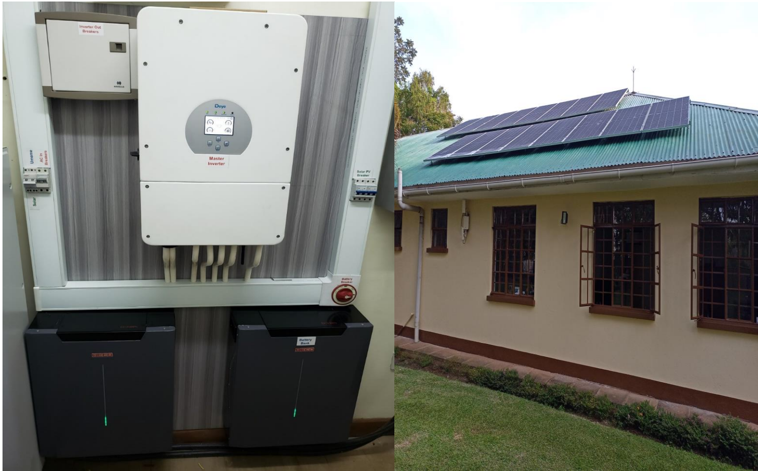
Below photo: Solar plant for Entebbe NIH block, the inverters and battery.
