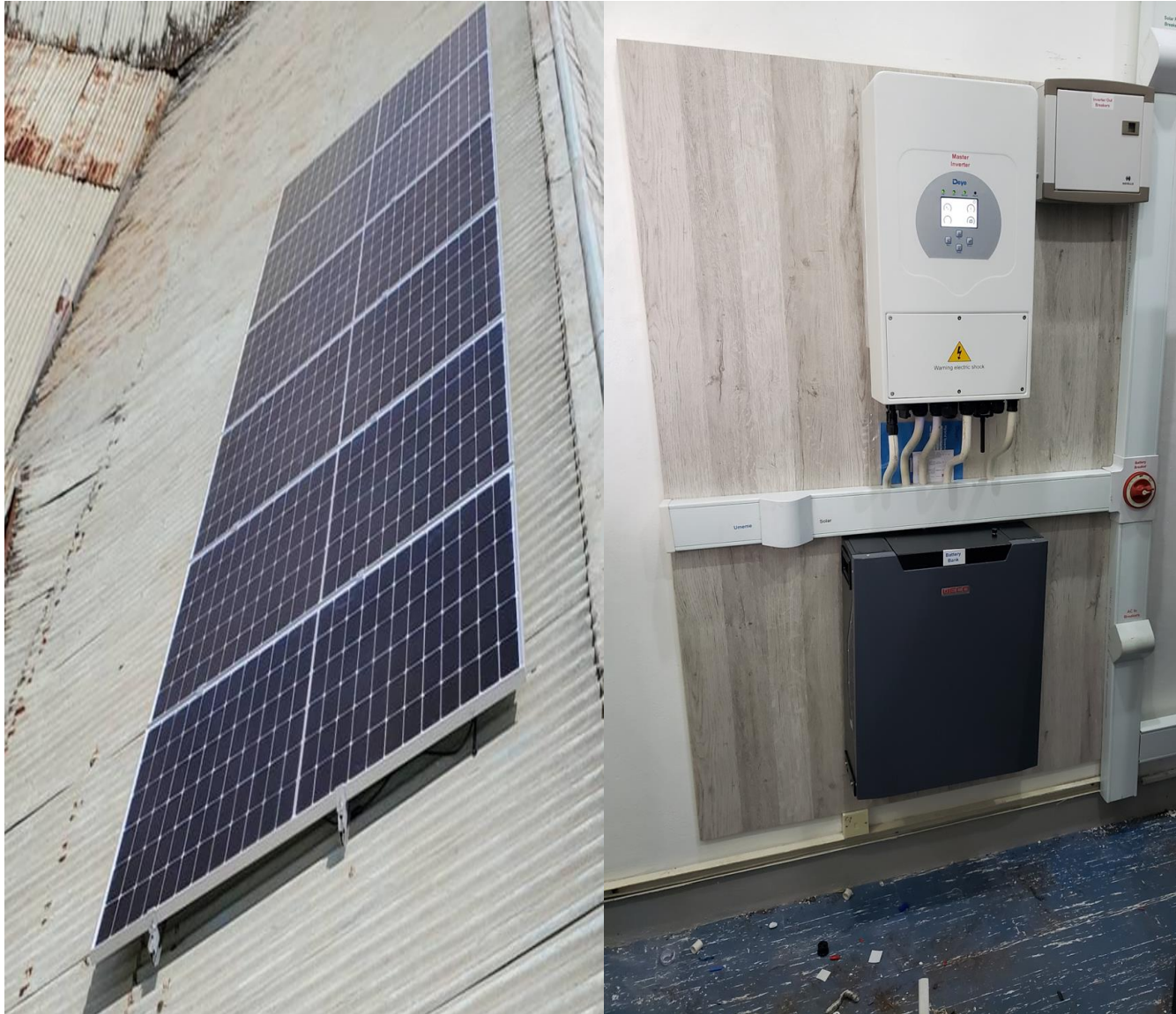
Photos below for Entebbe data Center and the solar installation feeding it.
