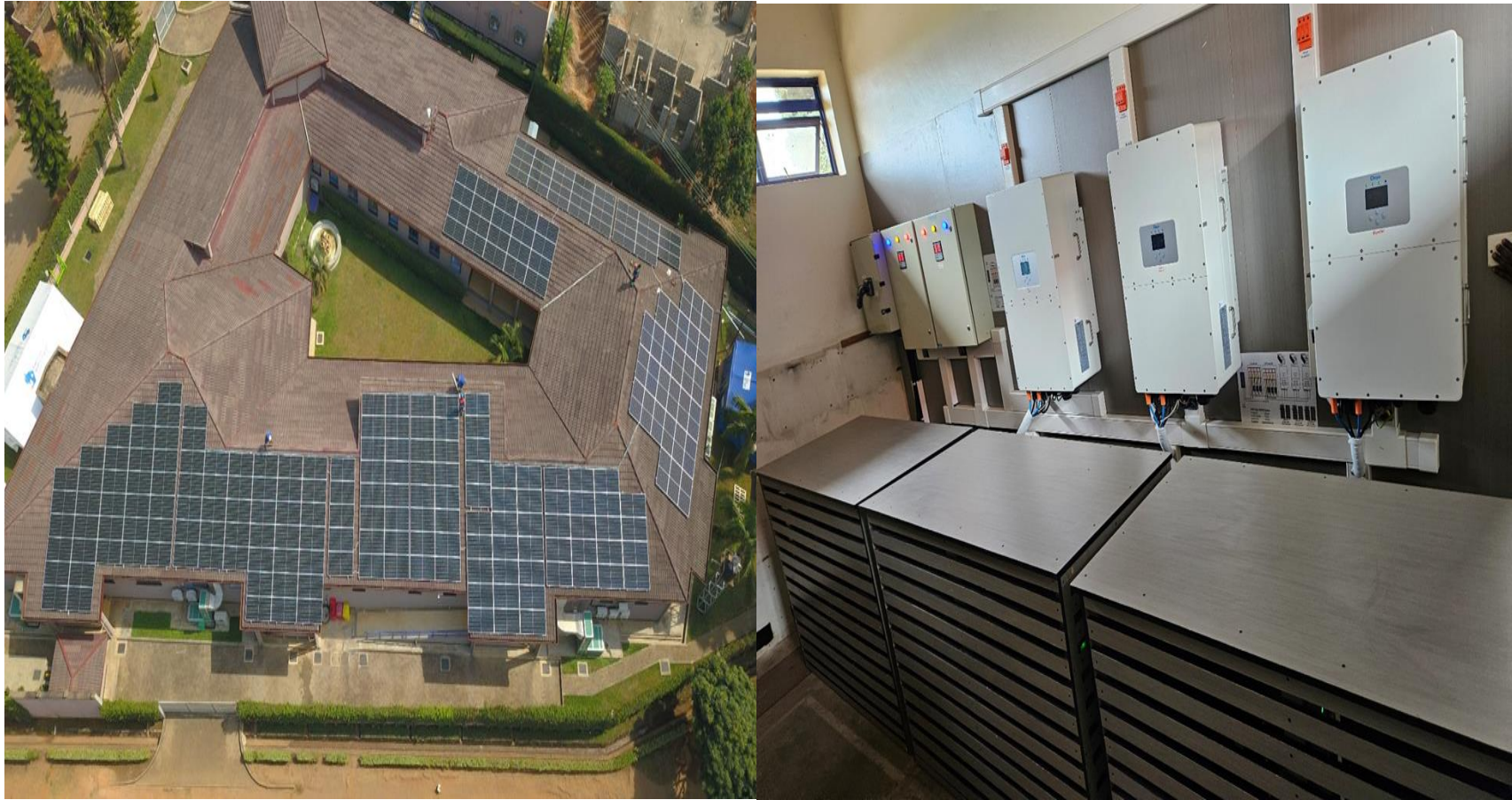
Photo above: Kalisizo field office Solar Installation
