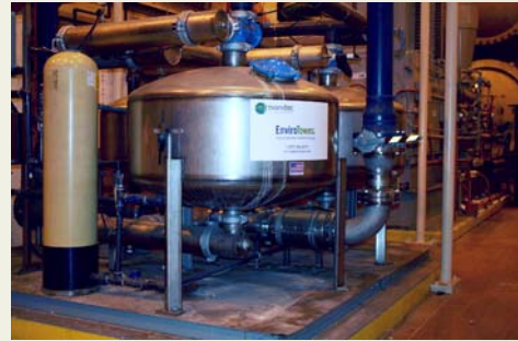
The Envirotower sits amongst the other media filters in Building 11.
