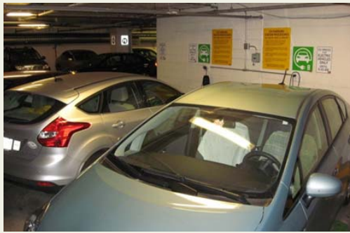
The underground parking garage that services the CRC is home to several electric vehicle charging stations.
